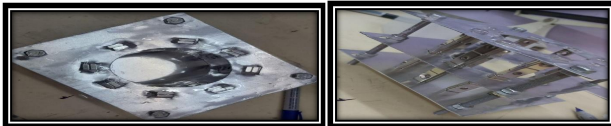
Figure (1): installation of the magnetic water device
